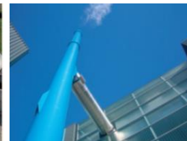
Flue gas treatment
